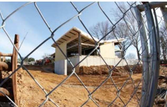
The new Lower School, under construction for most of this school year, will be completed in time for classes to begin in September.
